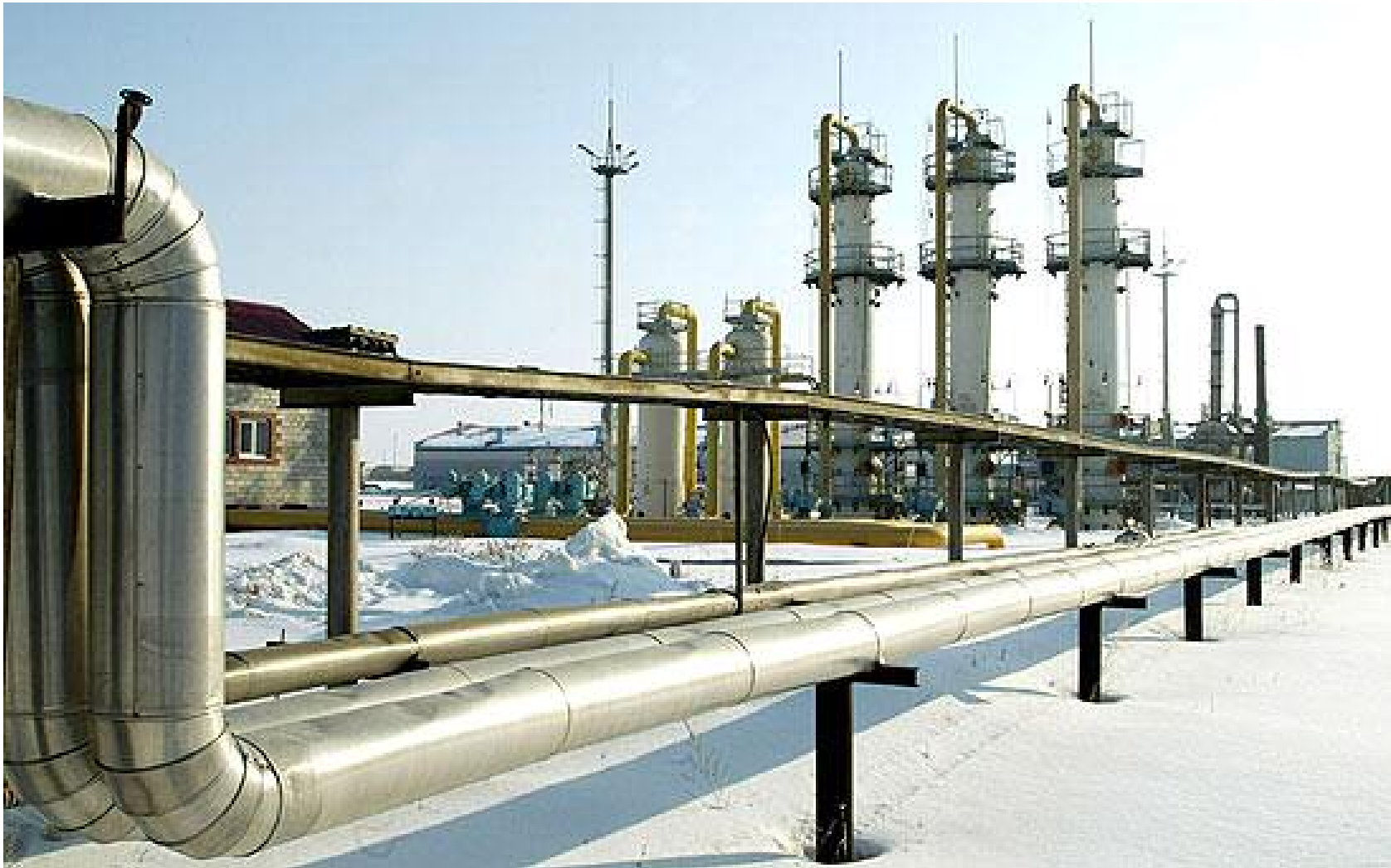
Gas Terminal and pipes.
