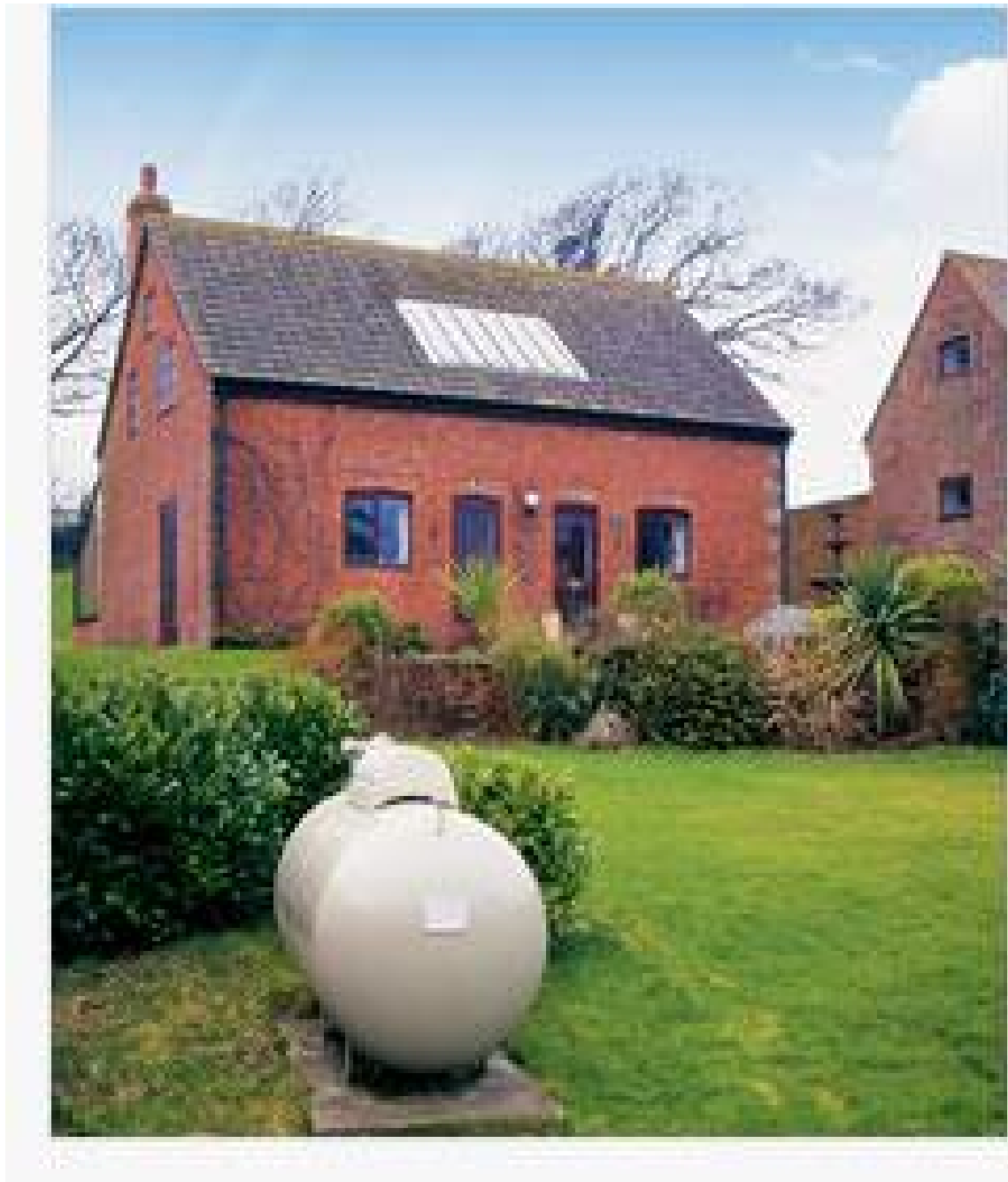
Domestic gas tank used for household central heating
