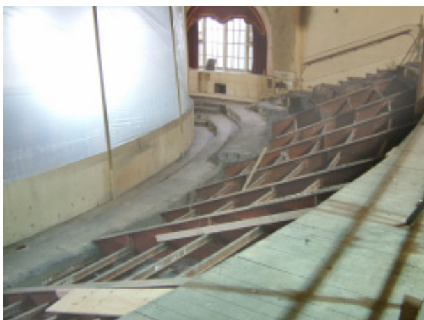
Removal of the original failed concrete to the Upper Circle nears completion behind protective screens. The original steel beams will be retained.
