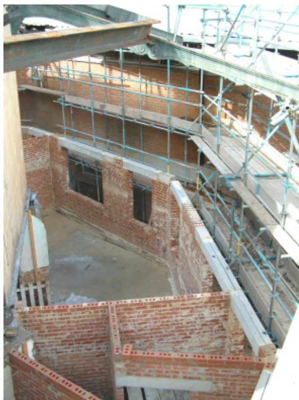
Following demolition of this structurally unsafe area, work is under way to provide new dressing rooms at the lower level, and restore the conservatory and ambulatory at the higher level. The ambulatory is the corridor encircling the building and this was originally used for 'promenading'. Reconstruction of this facility is a key feature for restoring the architectural integrity of the building.
