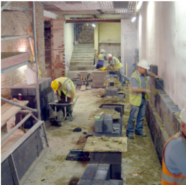
Construction work is underway to waterproof and stabilize the structure. This will be the location of the new toilets for ladies.
