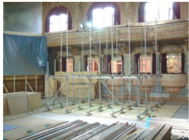
Scaffolding in the main auditorium to provide access for paint scrapings to be taken from the original ceiling. This is needed to establish the original decoration colours to ensure authentic redecoration. Floor protection and dust screens together with dust extraction systems are in place.
